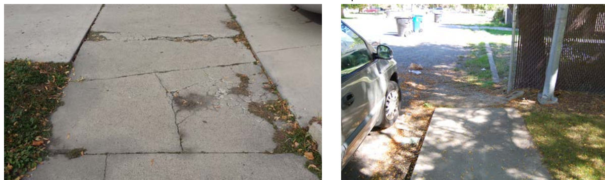
Figure 2.7 - Cracks and gaps in Franklin Neighborhood sidewalks
