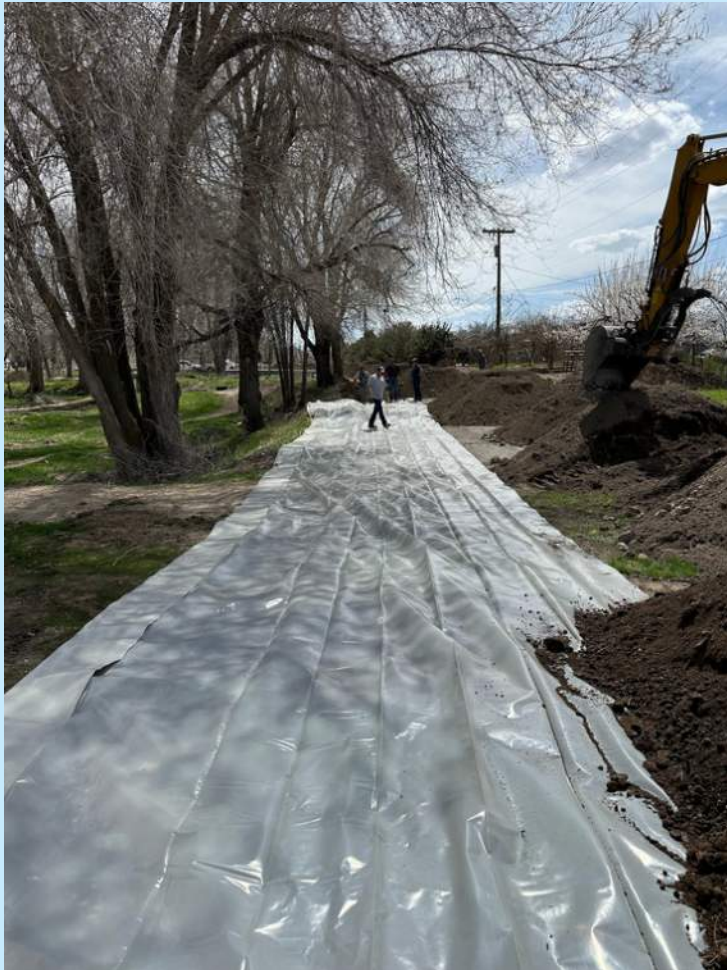
A berm was built in a high-risk neighborhood to block potential floodwaters.
